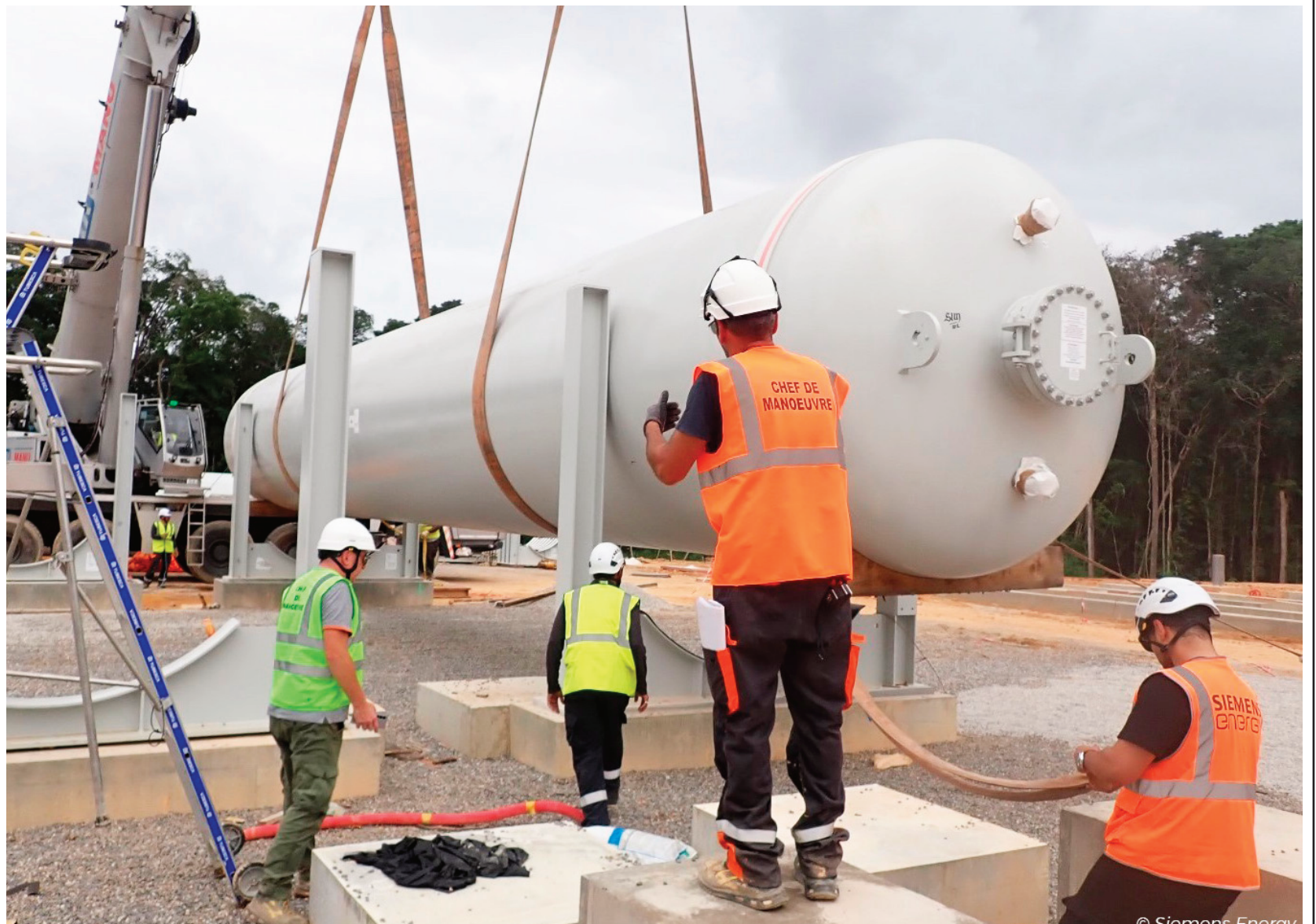
HYDROGEN TANKS INSTALLED on HDF’s pioneering Renewstable® plant in French Guiana. (GP)
